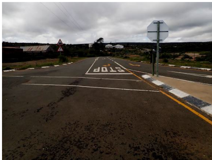
The recently sealed R335 at its junction with the R400 at Bracefield in the deep rural Blue Crane Municipality. A 15-km section of this gravel road has been sealed in a "tourism" project conceived and implemented by the Blue Crane Development Agency. The sealed section is in the middle of nowhere, extending from this junction 4 km north towards Somerset East and 11 km south to Anne's Villa. Photo: Richard Cowling
