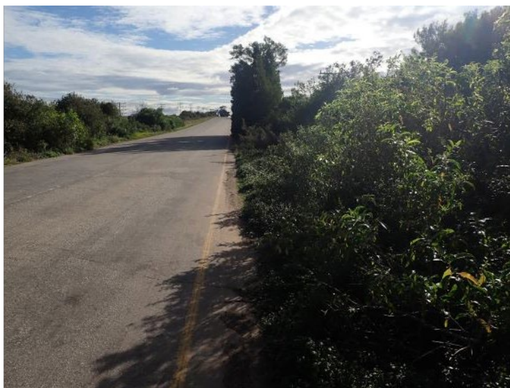
Overgrown verges along the R102, west of Humansdorp in the Eastern Cape. The Eastern Cape Department of Transport allocates zero funding for road verge maintenance in the western parts of the province. Photo: Richard Cowling
